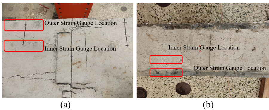
Fig. 9 Cracks on beam top surface: (a) RCB beam top surface, (b) UR-30-D8 beam top surface
