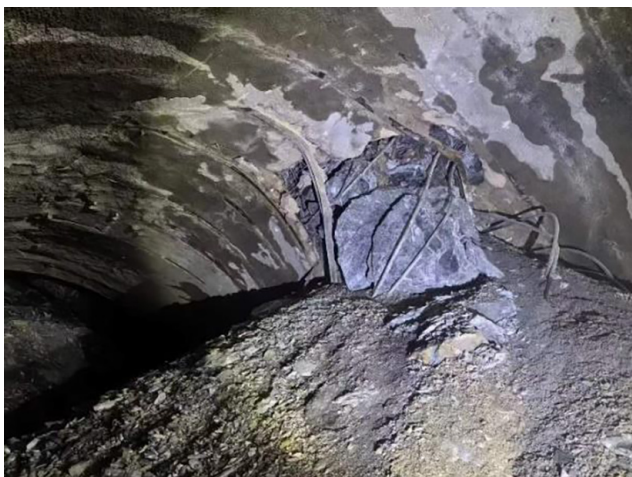
Fig. 1 The large deformation disaster of the tunnel primary support
