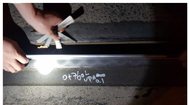
Fig. 4 Rail corrugation on line section 3
