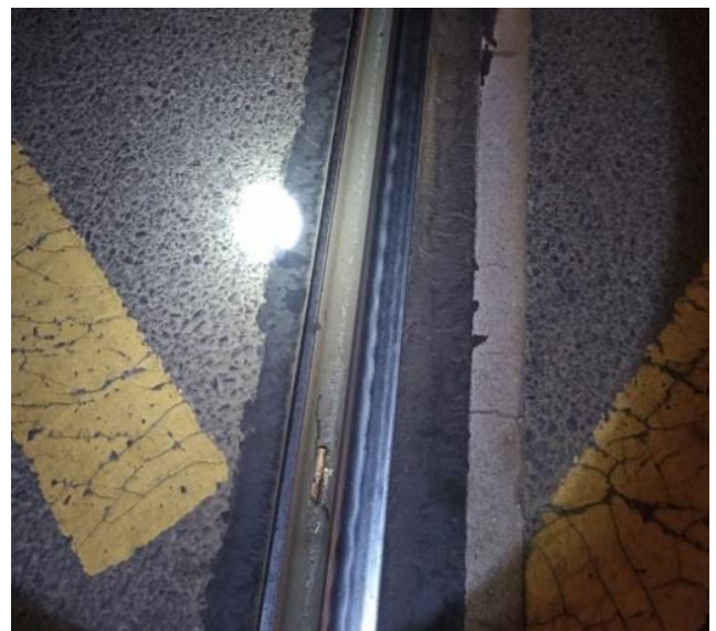
Fig. 3 Inner rail corrugation on line section 2
