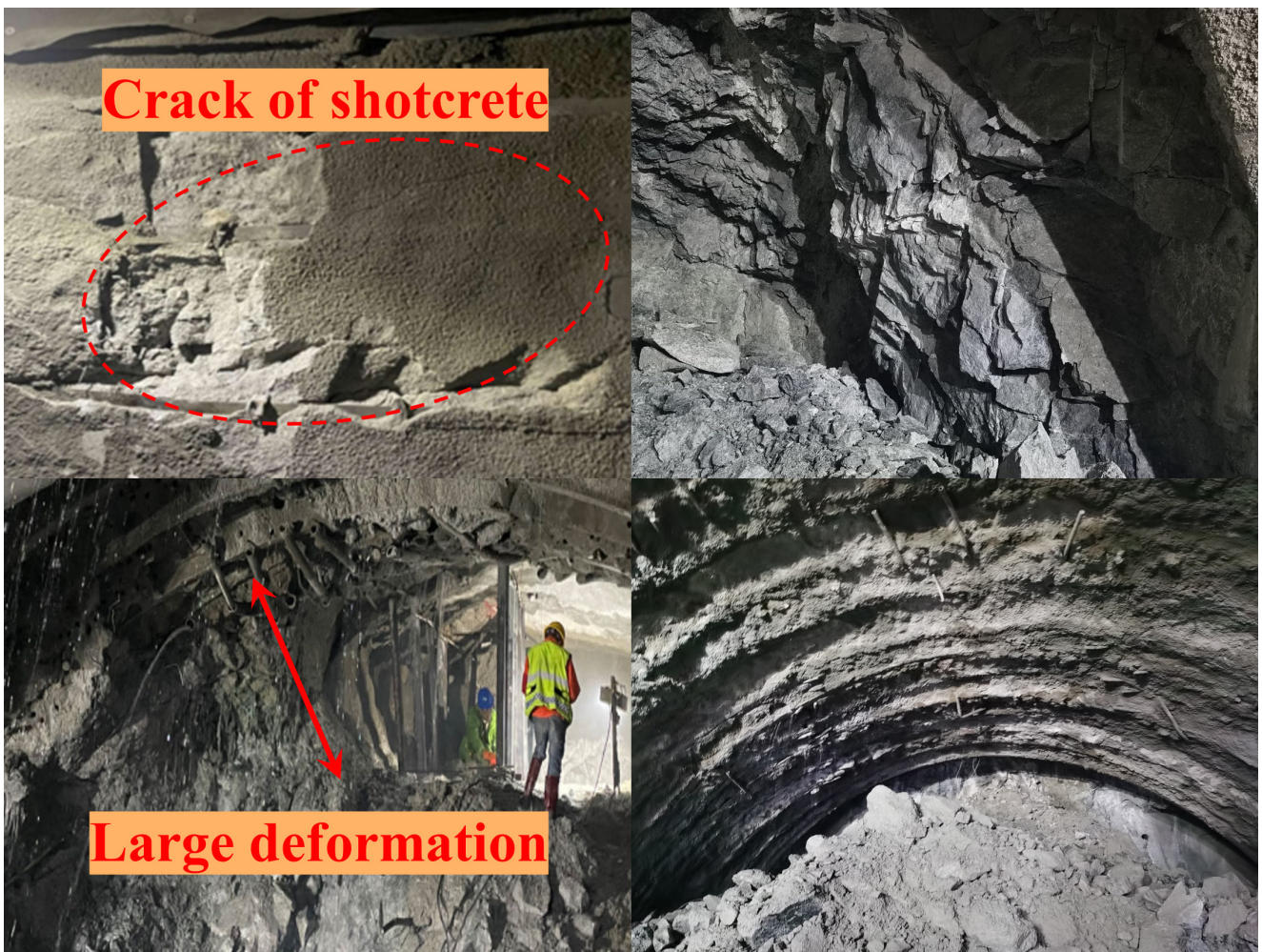
Fig. 1 The field rock layer joints and engineering disaster
