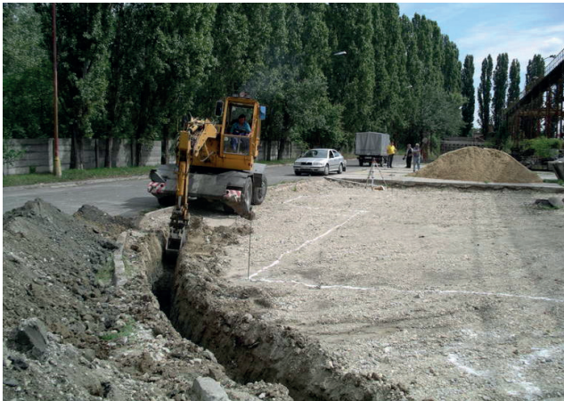
Fig. 20 Excavation for cooling circuits and heat recovery heat exchanger pipe-in-pipe with forced ventilation - outside the building at a depth of 2 m (Photo archive: Kalús, D.) [2]
