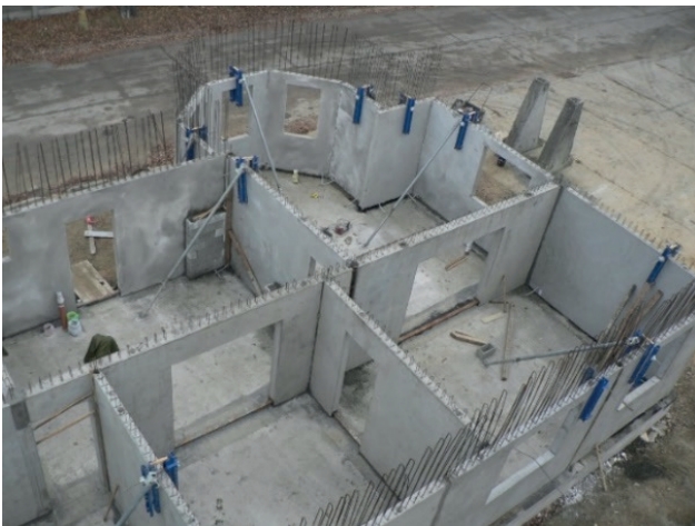
Fig. 5 View of the completed assembly of the ground floor (Photo archive: Kalús, D.) [2]
