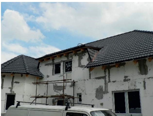
Fig. 9 View of the implementation of the insulation of the perimeter panels (Photo archive: Kalús, D.) [2]
