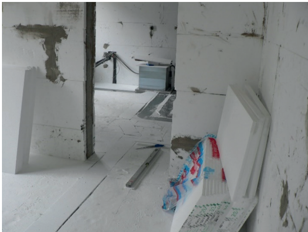
Fig. 8 Additional wall insulation also on the inside - the mass of the building walls, including the interior walls, serves as a large-capacity heat/cooling reservoir (Photo archive: Kalús, D.) [2]
