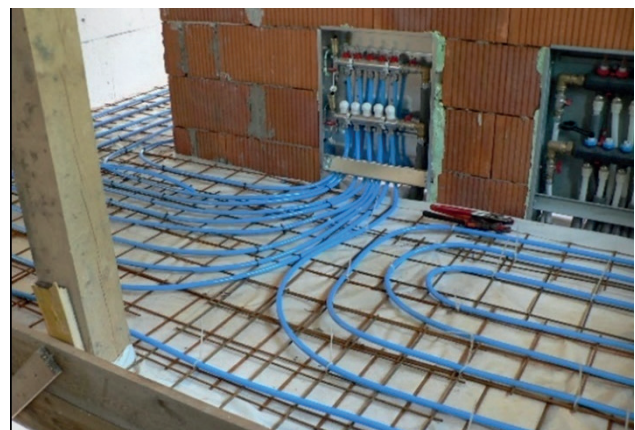
Fig. 16 View of the distributor and collector of the underfloor heating (Photo archive: Kalús, D.) [2]
