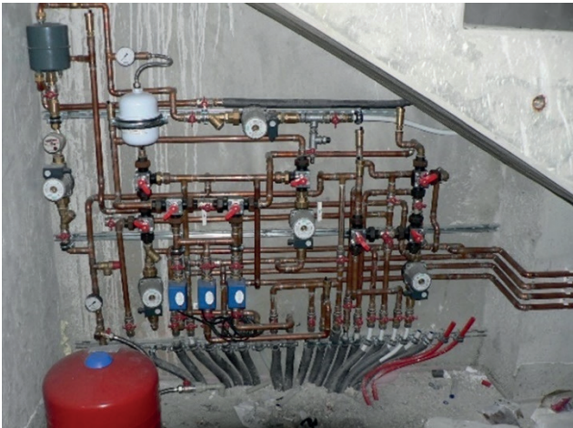
Fig. 17 View of the complex connection of the combined building-energy system (Photo archive: Kalús, D.) [2]
