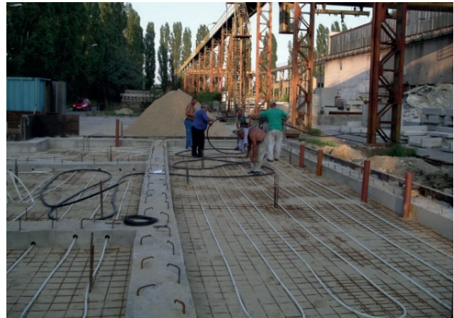
Fig. 21 Installation of piping system for preheating hot water (Photo archive: Kalús, D.) [2]
