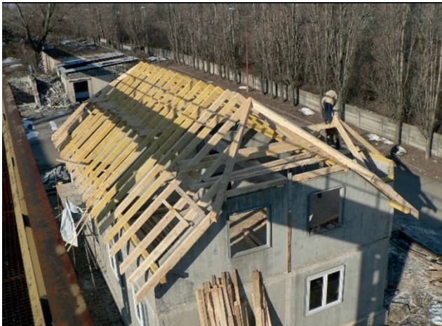
Fig. 7 View of the realization of the wooden truss (Photo archive: Kalús, D.) [2]
