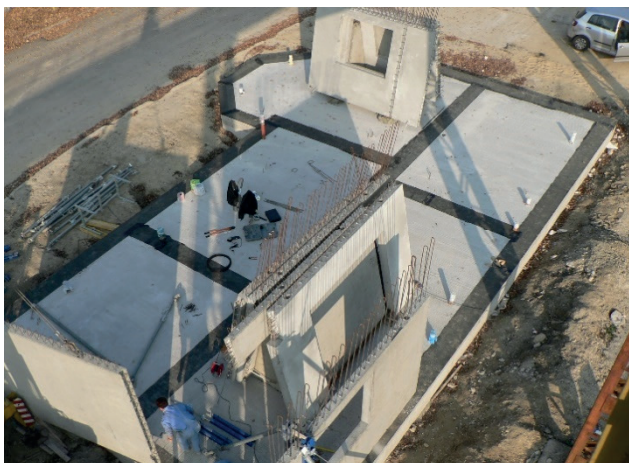
Fig. 26 A view of the beginning of the installation of panels with integrated energy-active elements in the function of a thermal barrier [2]
