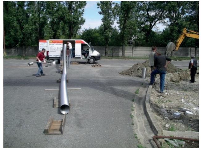
Fig. 18 Fabrication of the stainless-steel pipe-in-pipe heat exchanger on site (Photo archive: Kalús, D.) [2]
